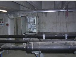
400 kV cable joints
