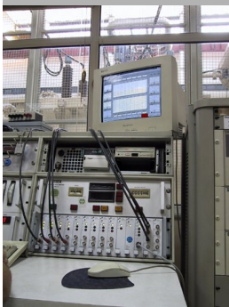
HV control room
